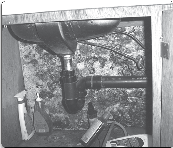
Plumbing leaks can lead to mould
