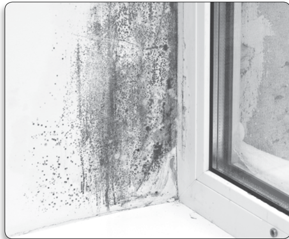
Mould can grow on damp drywall
