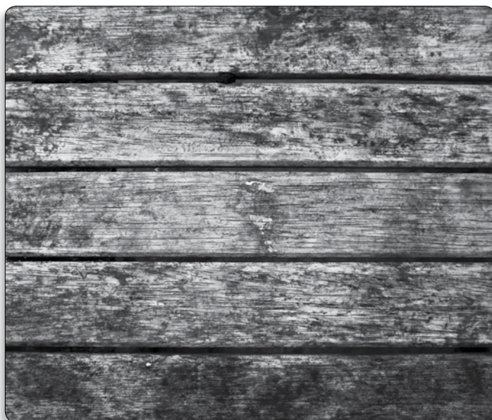
Mould growth can lead to wood rot
