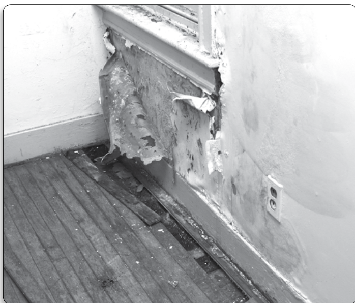
Water can lead to mould and can damage building materials
