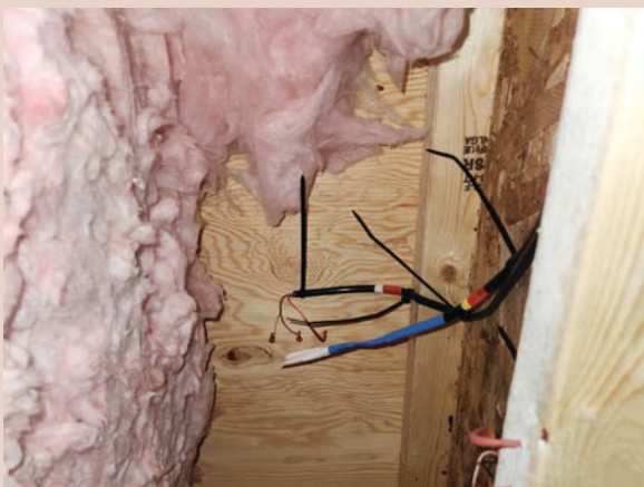
From top to bottom: Sanirajak community housing, photograph; split-insulated wall assembly, diagram; enclosure monitoring system installation at Sanirajak, photograph, Bawating Building Science.
