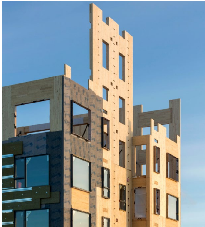
Figure 7. CLT panels used as exterior wall structure on the Origine building (Cecobois, 2018) (courtesy of Stephane Groleau).
