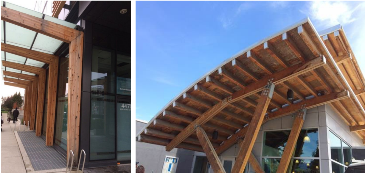
Figure 11. A canopy (left) and a roof overhang (right) used to protect exterior wood members.
