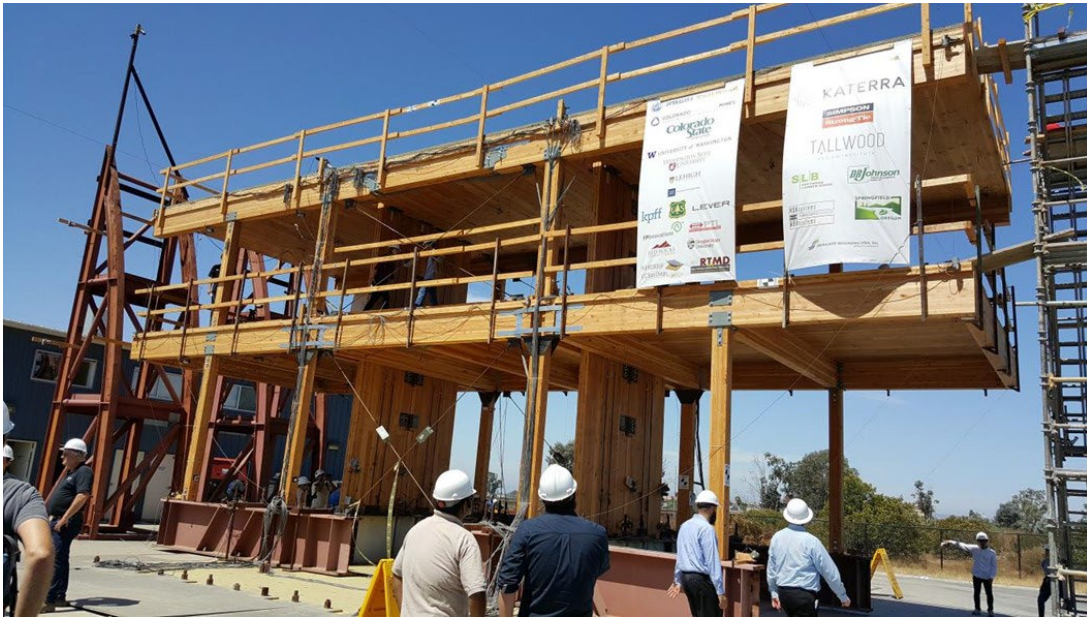
Figure 40. Full-scale 2-storey CLT building tested at the shaking table, University of California San Diego.
