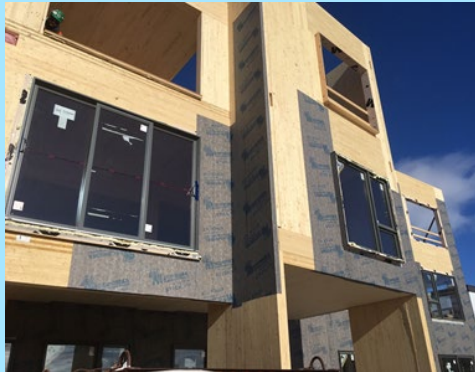
Mass timber construction using CLT panels with self-adhered air barrier membrane installed on the exterior surface.
