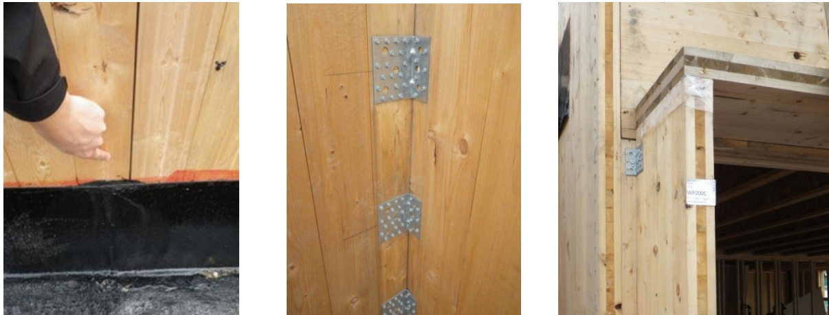
Figure 12. Some of the unique air barrier detail considerations required for CLT panel assemblies when used within tall wood buildings: gaps between lumber plies and connections (left), structural anchors interfering with installation of the air barrier membrane (centre), and protruding structural elements (right).
