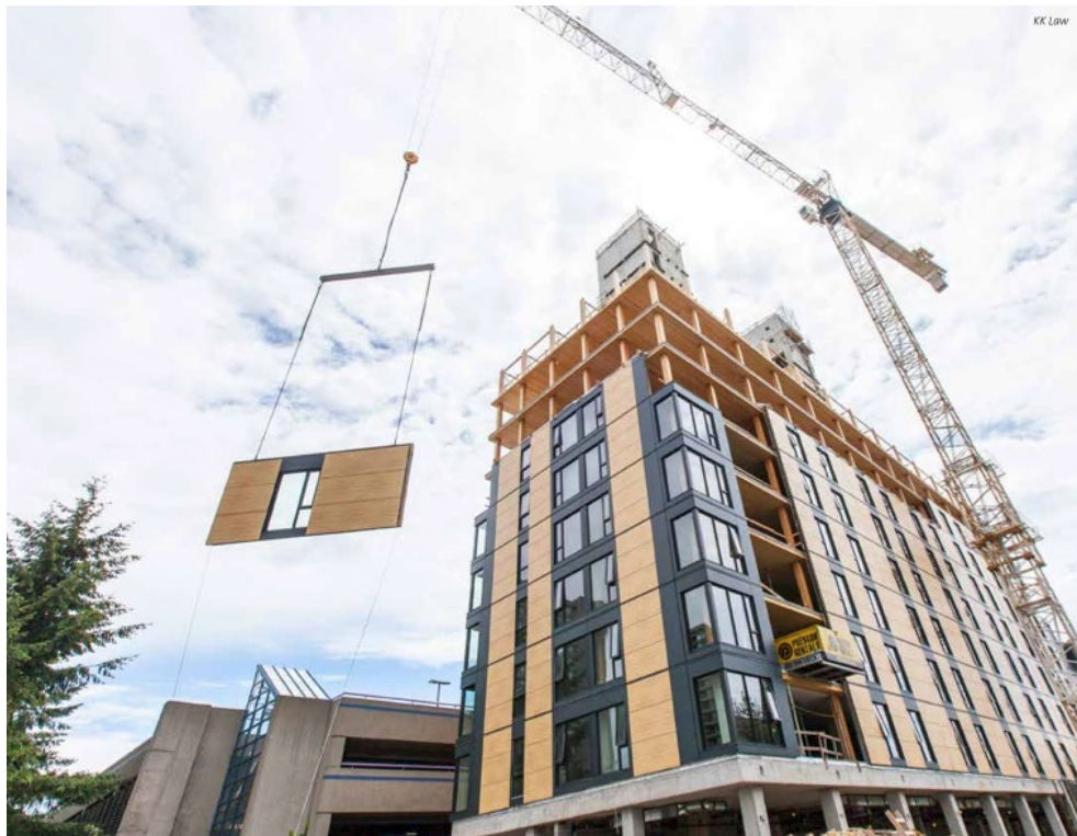
Figure 2 Brock Commons envelope installation within 2 storeys of “live” structure floor (UBC, 2016) (courtesy of KK Law).
