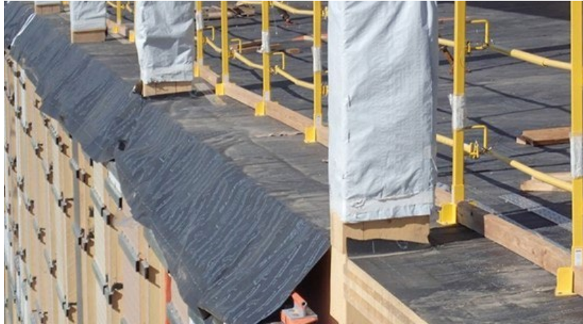
Figure 17. Vapor-permeable WRB over CLT floor panels is draped over the wall system below to shed water away from the lower levels of the building.
