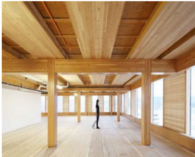
Figure 12. Plywood furring used to create an air space between plywood roof sheathing above and CLT panels below, in the Wood Innovation and Design Centre, Prince George, B.C. (courtesy of Michael Green Architecture).
