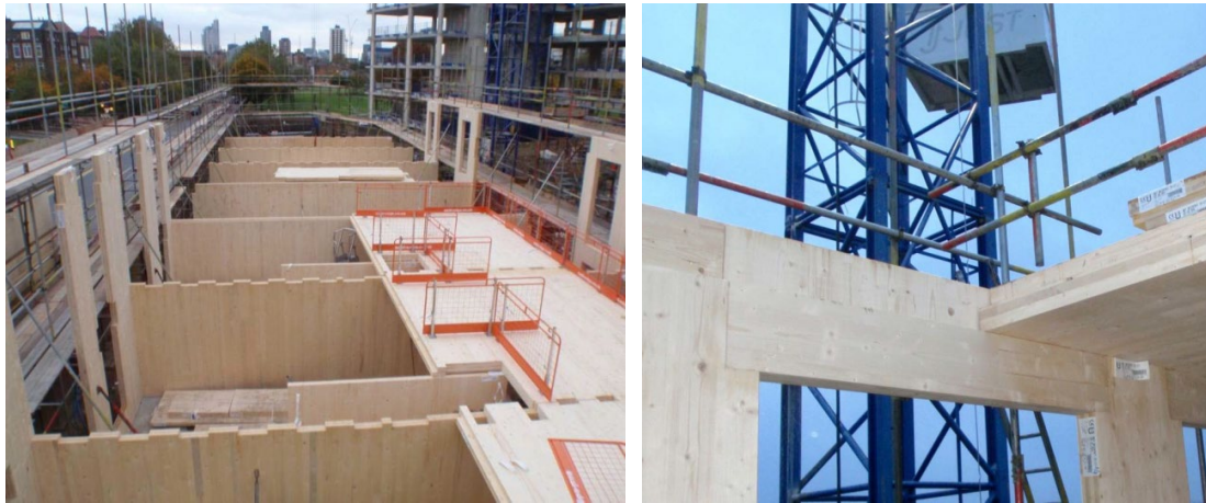
Figure 5. Minimizing compression perpendicular to grain and shrinkage using profiled panel ends (courtesy of Eurban).
