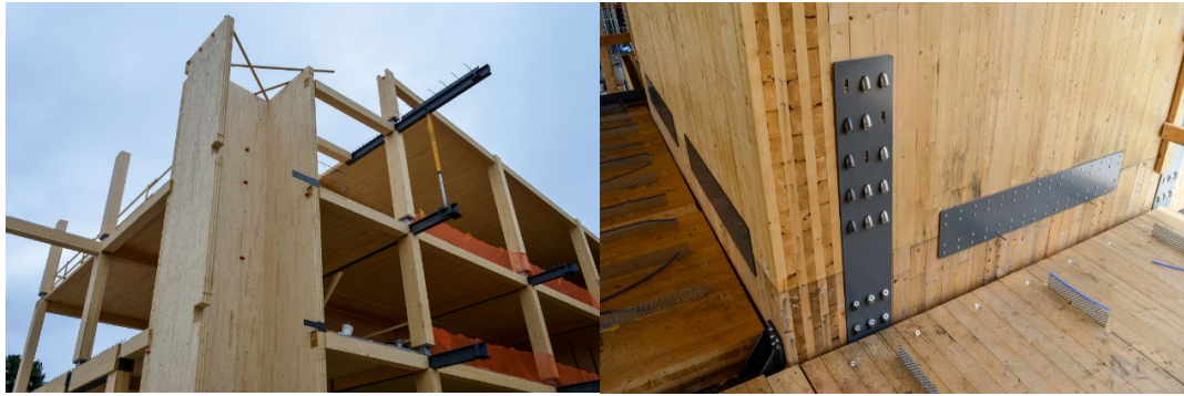
Figure 17. Shearwalls and details, University of Massachusetts, John W. Olver Building (courtesy of Alex Schreyer/ University of Massachusetts).
