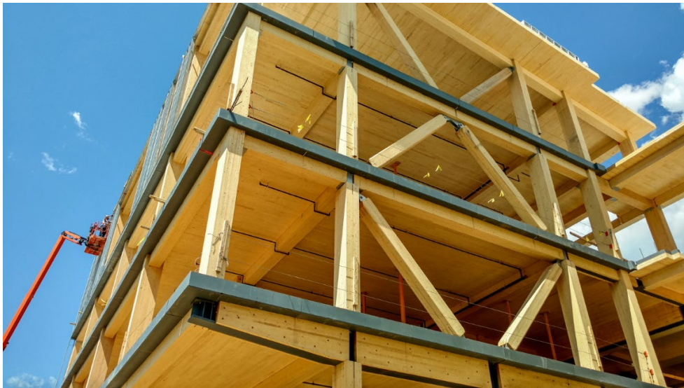
Figure 19. Timber bracing, University of Massachusetts, John W. Olver Building (courtesy of Alex Schreyer/University of Massachusetts).
