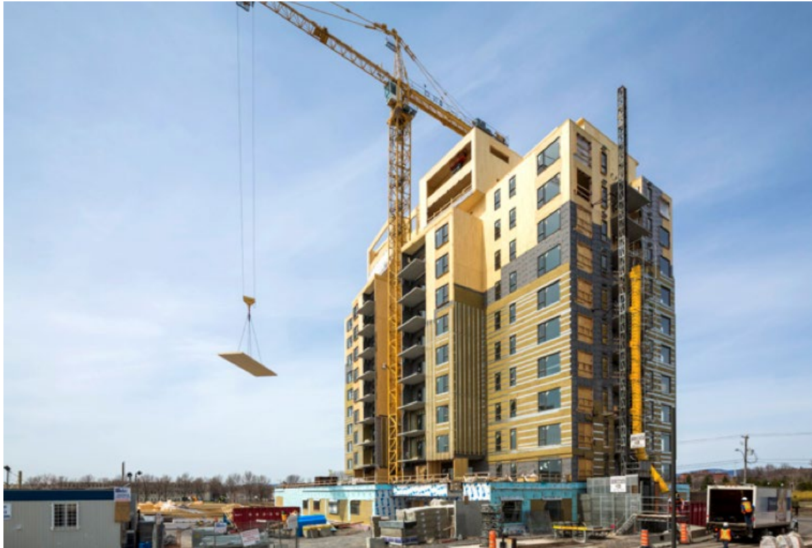
Figure 6. Lifting the last panels to complete the Origine structure (Cecobois, 2018) (courtesy of Stephane Groleau).
