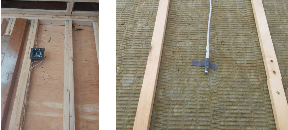
Figure 7. Small sensors installed to measure the service environment and performance of wood-frame construction (left: a relative humidity/temperature (RH/T) and moisture pin sensor installed on the interior side of plywood sheathing; right: an RH/T sensor installed in the rainscreen cavity to measure the exterior environment).
